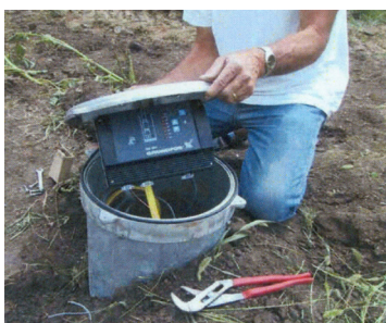
Control mounted on plate attached to lid
