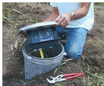
Control mounted on plate attached to lid
